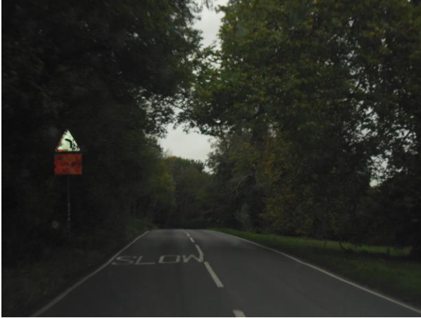
Image 3 – View travelling northbound on Coopersale Street before bend. Bend warning sign is in poor condition.
